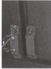
Figure 48. Magnetic switch on a sliding door.
